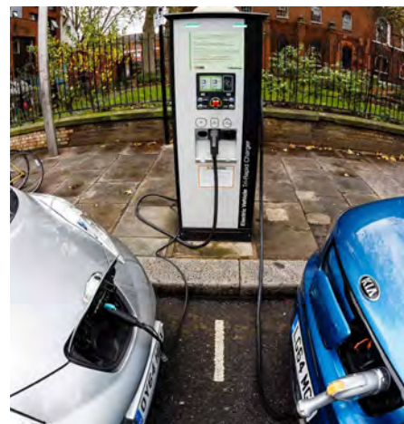
Electric vehicle charging points
